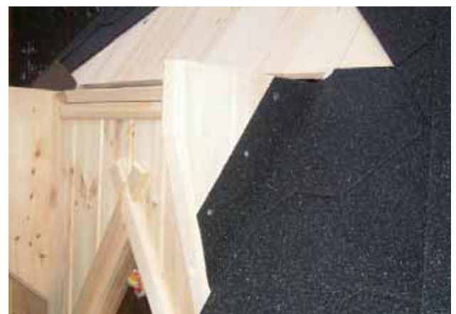
40. Turn the roofing material up against the casing and cut it to make it neat.
