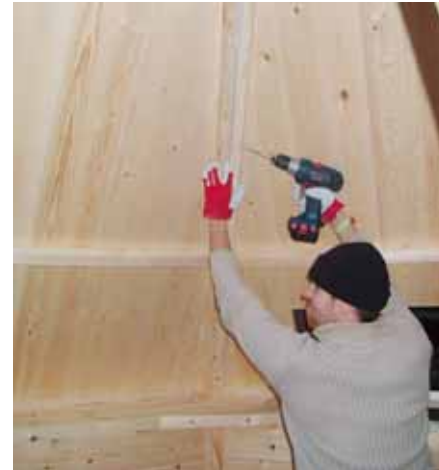
28. Screw the roof elements together immediately after you raise them up (6 x 80).
