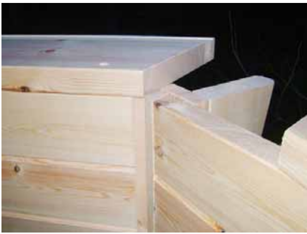
9. Begin from the back wall by placing a ledge even with the corner of the wall.
