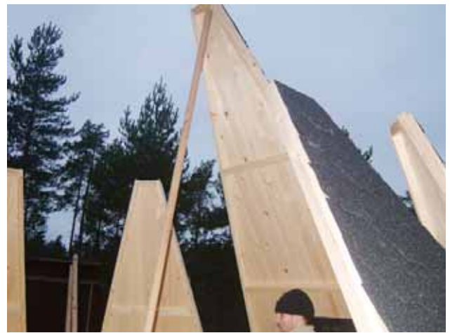
26. Raise the roofs one at a time; use the three 3.5-meter props to help you.
