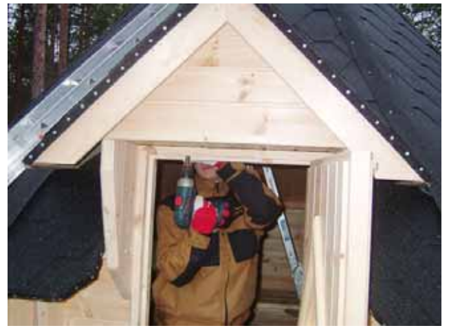
42. Lift the small roof over the door and fasten it through the frame (6 x 80).
