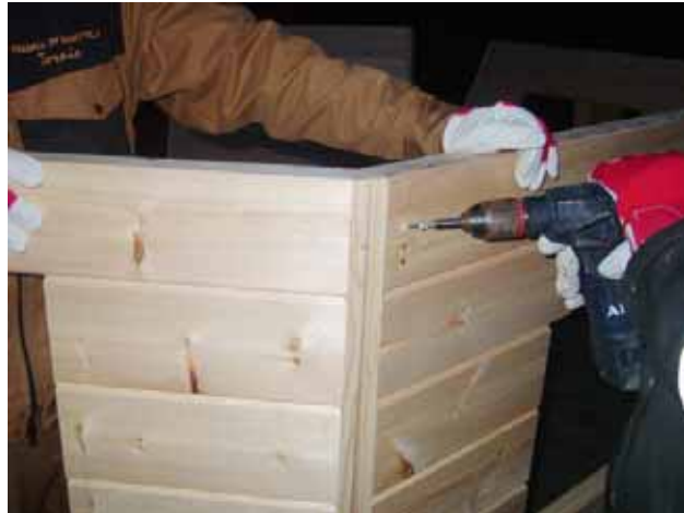
3. Make sure the top parts of the walls are even with each other.
