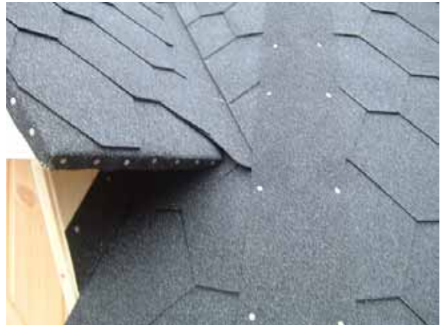
46. Cut the roofing on the small roof and nail all of the edges, including the roof over the door.
