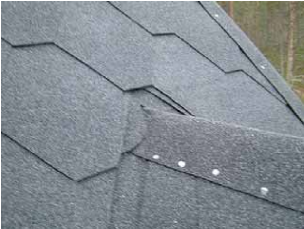
45. Put a piece of roofing on the upper corner of the small roof to prevent water from getting inside.
