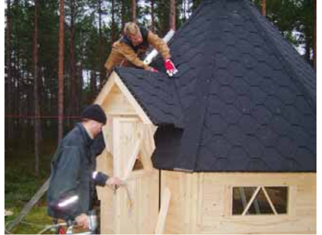
44. Make sure the roofing on the small roof goes under the roofing on the pavilion roof.
